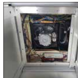
A5. Condenser compartment
